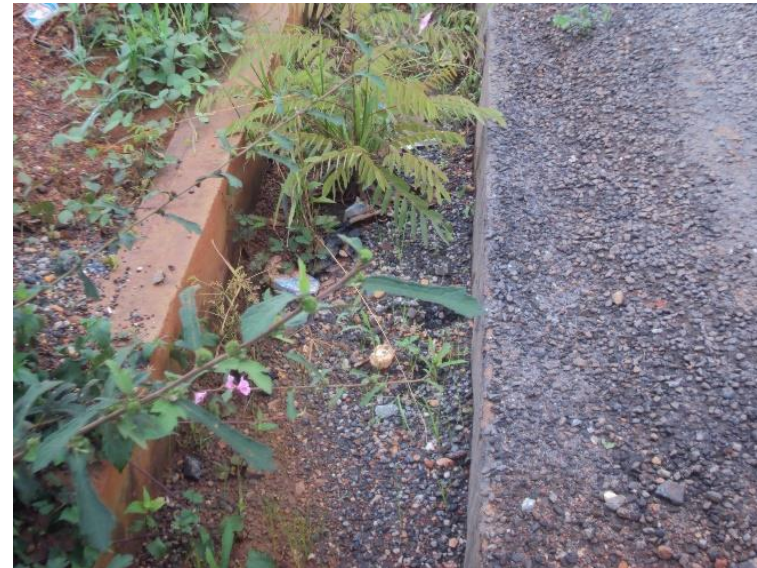
Plate 3a: Drain filled with soil, weeds
