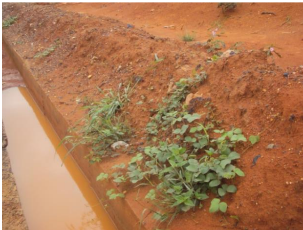
Plate 3d: Eroded soils and debris into drain
