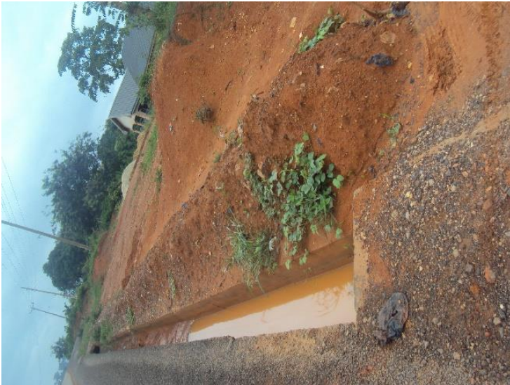
Plate 3e: Too steep banks of constructed drain
