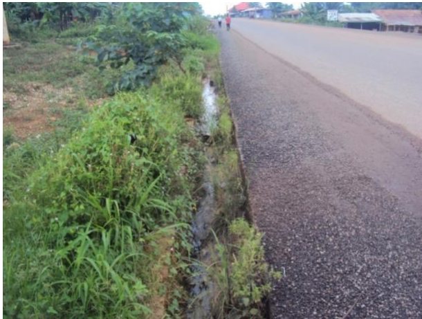
Plate 3c: Deactivated drain use as weeds continues to grow in drain with settled water
